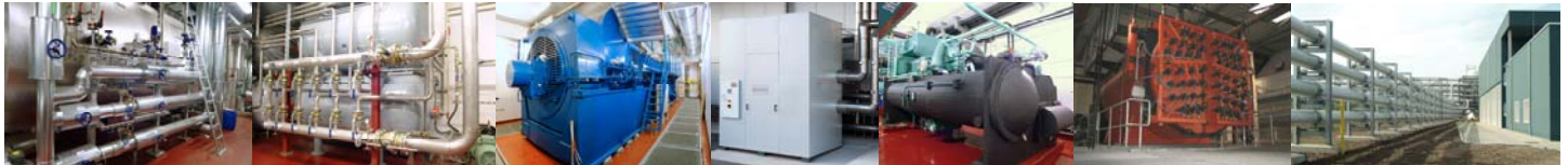
steam boiler compressed air distributor CHP motor ago congelo chiller combustion chamber energy bridge
