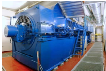
Gas engine of a combined heat and power plant
