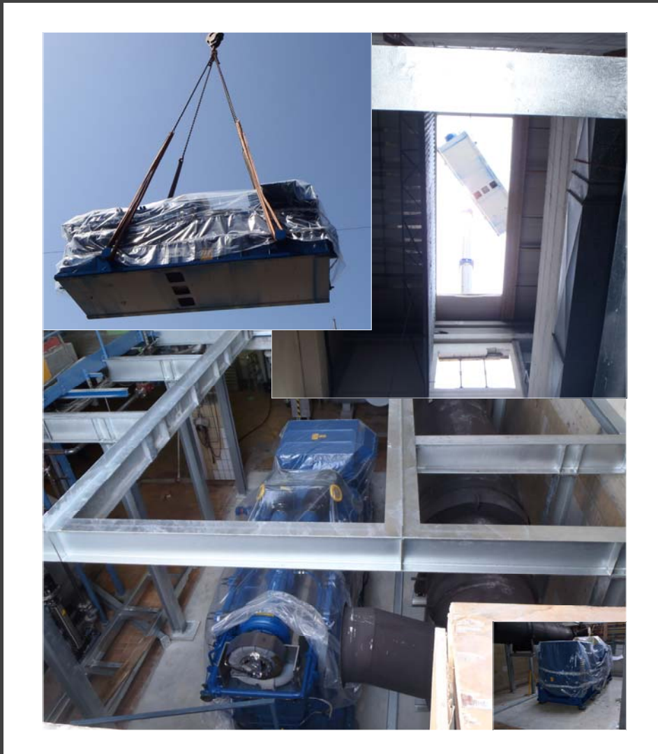
Positioning and adjustment of the aggregate with a capacity of 1.5 MWel, as well as installation
